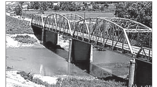
View of the three types of truss components of the Hazelgreen bridge.
